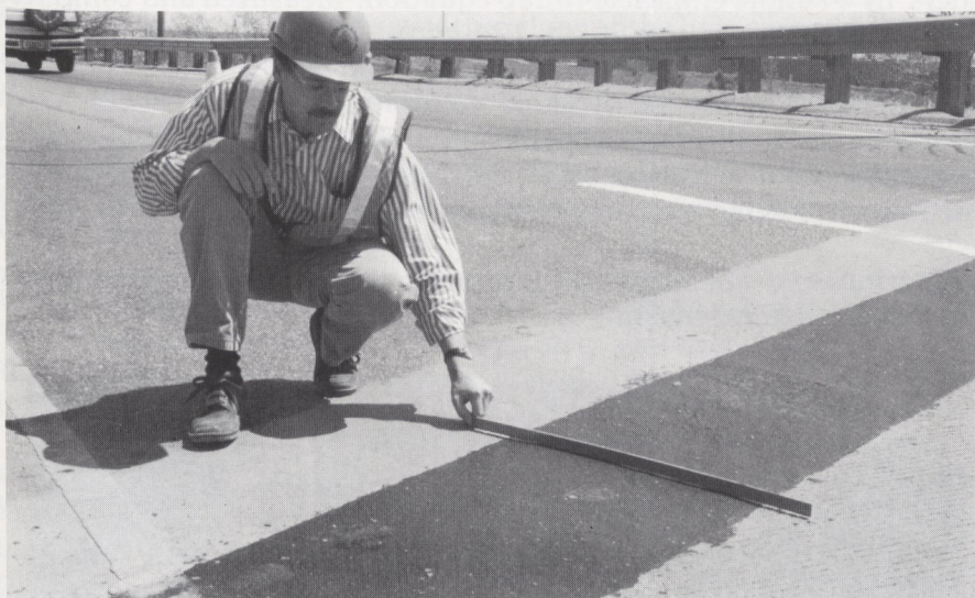
David Woodham, Research Branch Engineer, checks the level of a newly installed Koch Bridge Joint System.
